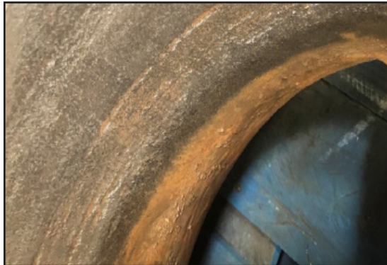
Severely damaged suction bell before repaired with ARC 858 .
